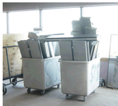
<< Carts filled with ductwork removed during a renovation at Boston Scientific in Marlborough, Massachusetts.
